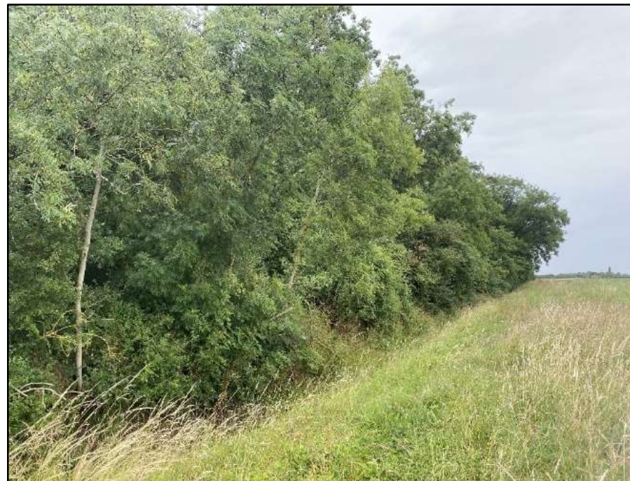
Location: 28 NGR: TF 14133 48209 Photo Date: 14 July 2023 Description: Unnamed drain, with hedge and overgrown vegetation throughout channel, left bank c.1.5m, right bank c.1.5m, width c.2m. Facing north.
