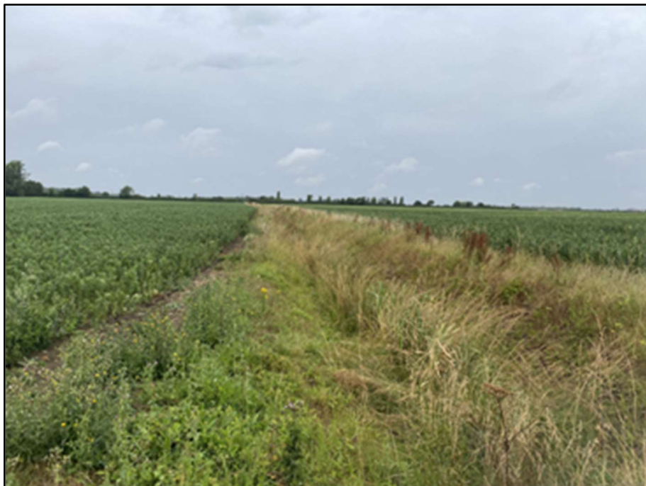
Location: 27 NGR: TF 14140 48279 Photo Date: 14 July 2023 Description: Unnamed drain, with hedge and overgrown vegetation throughout channel, left bank c.1.5m, right bank c.1.5m, width c.2m. Facing east.
