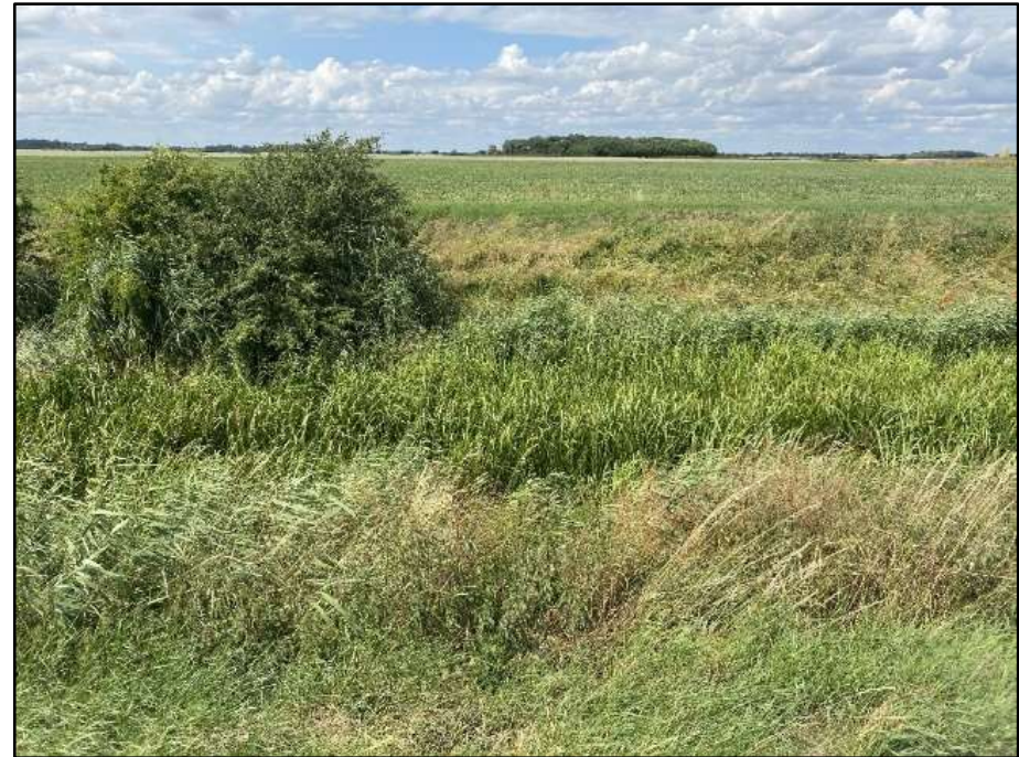
Location: 12 NGR: TF 15111 47772 Photo Date: 13 July 2023 Description: Hodge Dike, overgrown vegetation throughout channel, left bank c.2m, right bank c.2m, width c.5m, channel c.0.3m. Facing north.
