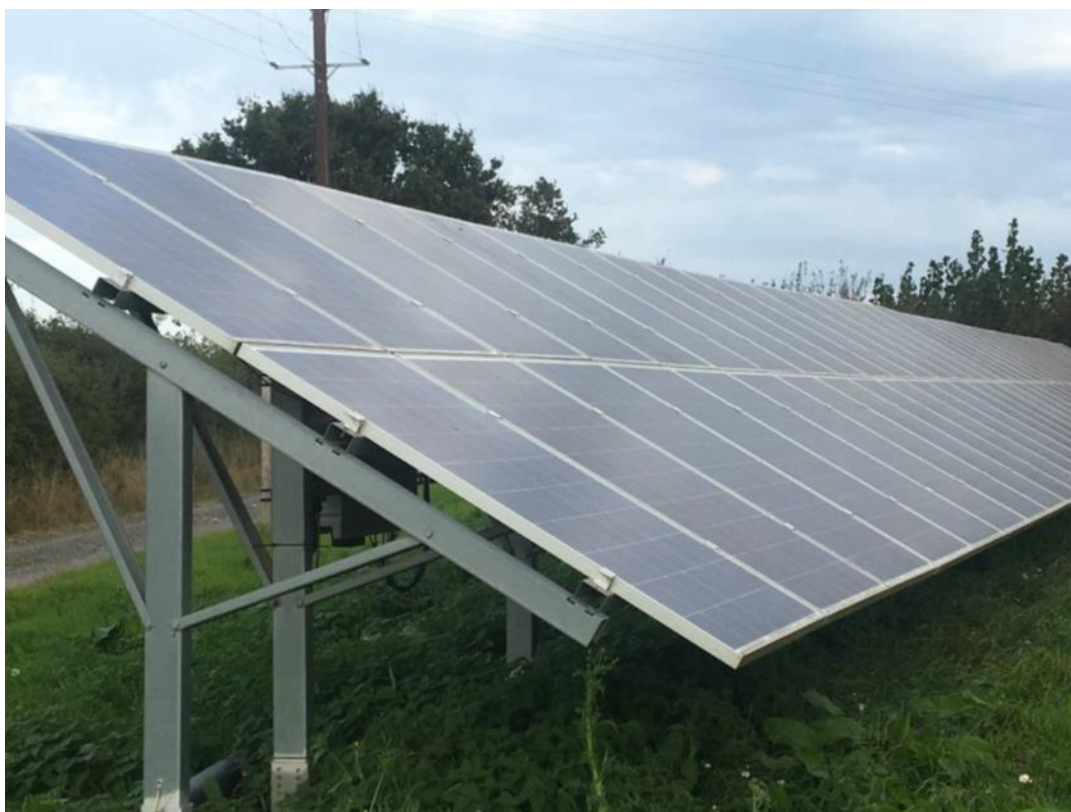
Figure 2.1 Solar panels with south facing configuration.
